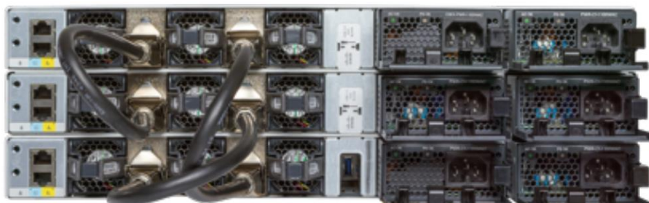
Figure 5. Cisco Catalyst 9300 Series switch stack units
